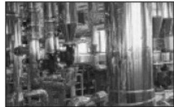
Industrial applications Courtesy UMDE Engineering, Contracting, and Trading. Used by permission.
