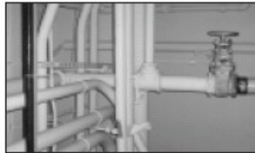
Piping and plumbing systems Photo by John M. Cimbala.
